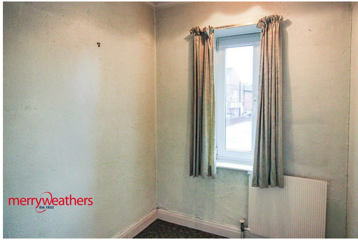
Front UPVC Window and central heating radiator.
