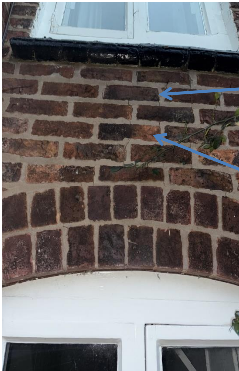
Settlement vertical cracks
